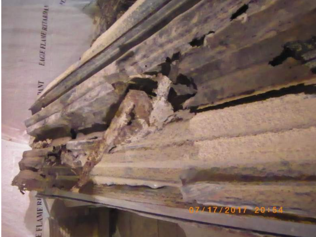
Figure 3. Corrosion damaged metal deck after removal of concrete.
